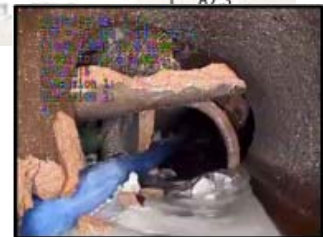
FIGURE 342A: CCTV IMAGE OF FIBER OPTIC CABLE CONFLICT
